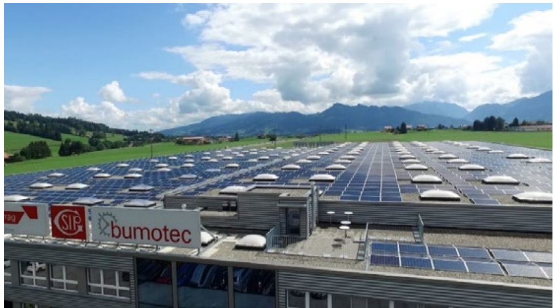
Solar installation on our manufacturing plant in Vuadens, Switzerland, that covers about 40% of the local electricity consumption
